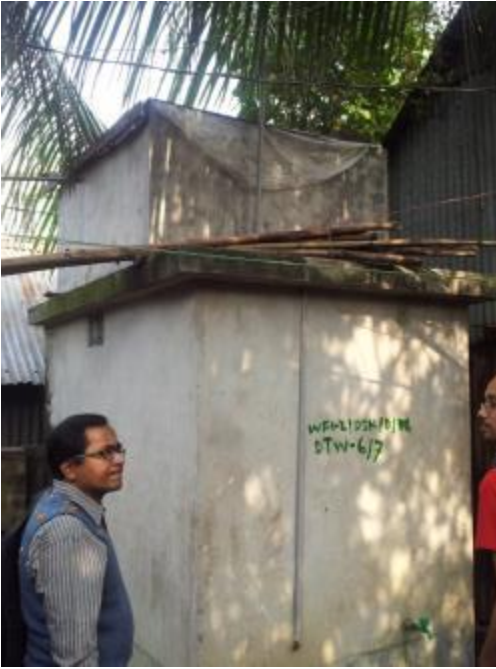
Community storage tank built by brick
