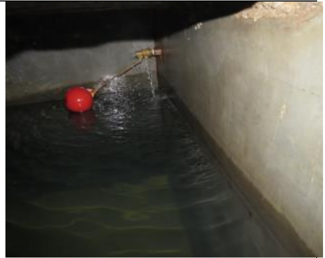
Valve control at the storage tank
