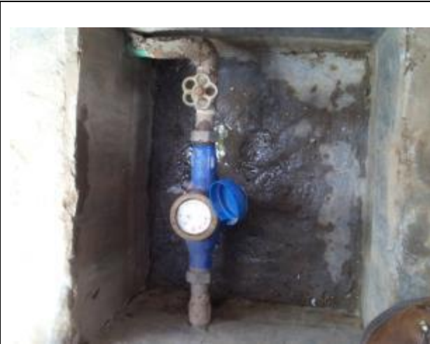
Water meter at the entrance of the storage tank
