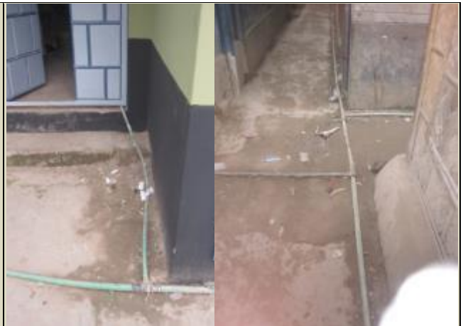
Household Piped Water Connection System
